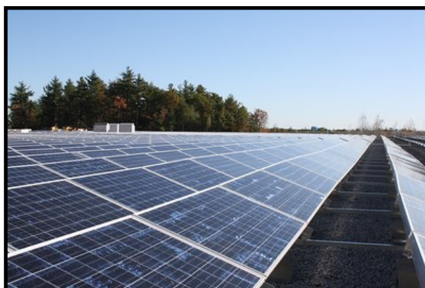
Westford (MA) Solar Park Photo credit: Office of Energy & Environmental Affairs
